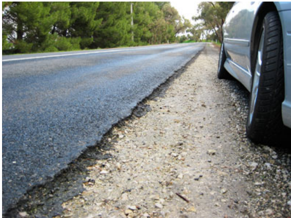
Photo 1 - Broken and dangerous road edge drop offs.
